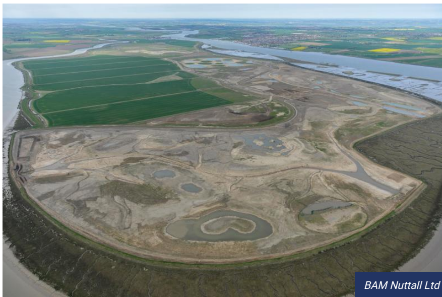
77. Construction of Jubilee Marsh, Wallasea Island, April 2015. This photo was taken prior to the introduction of tidal flooding. The pale
